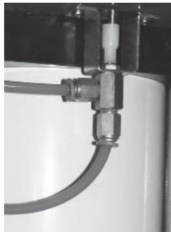
DOOR SAFETY SWITCH LOCATED BESIDE AIR CYLINDER ON THE UCC840C
